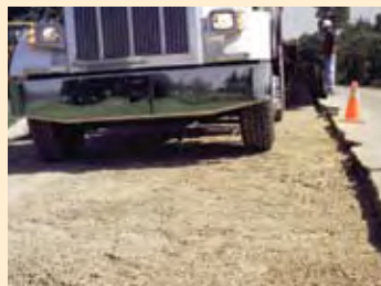
One hour after pouring, 4F Base is strong enough to support a 32-ton vehicle.
